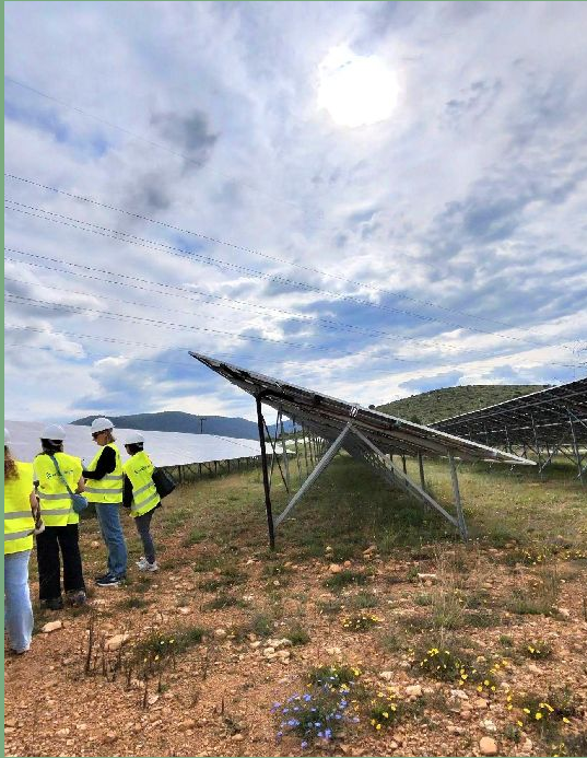
The Vasileiada PV Plant
