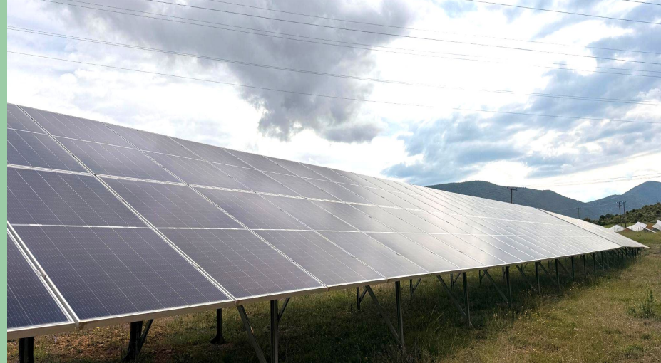
Vasileiada PV Plant, Western Macedonia
