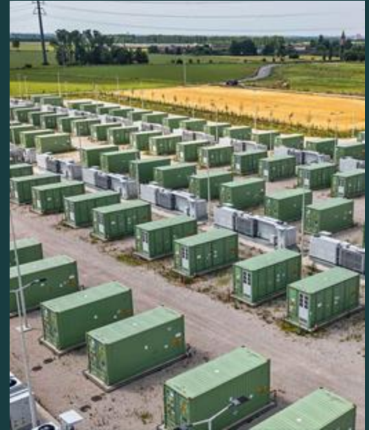
Battery energy storage systems, enel group
